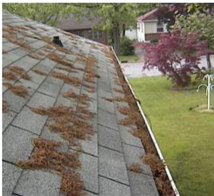
Improperly maintained gutters are habitats for nuisance and vector mosquitoes.
