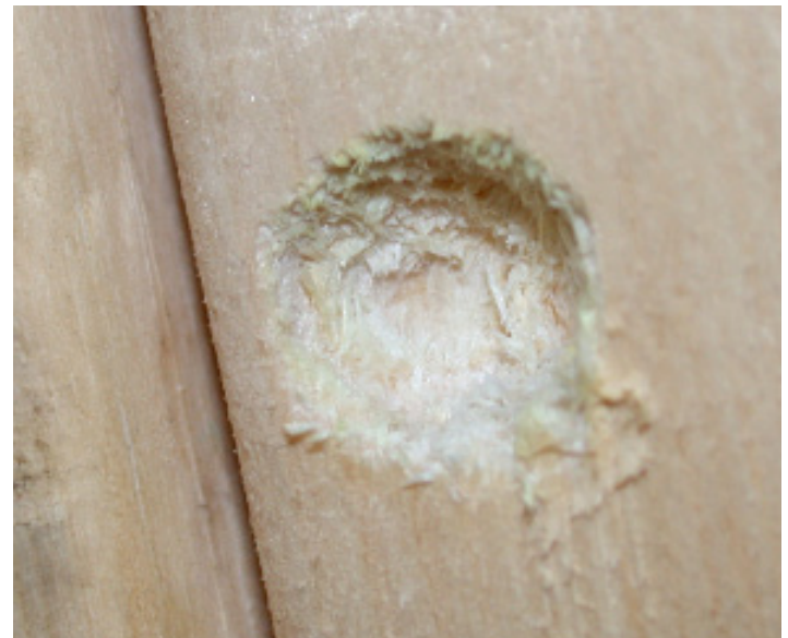
Beginning of hole that will eventually become nearly perfectly round and approximately ½ inch in diameter. (Photo credit: John Obermeyer)
