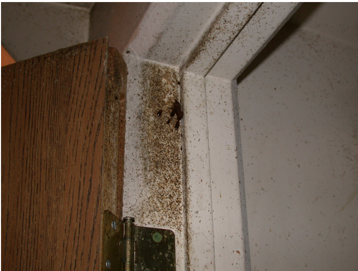
Signs of heavy cockroach infestations. (Photo Credit: Changlu Wang)
