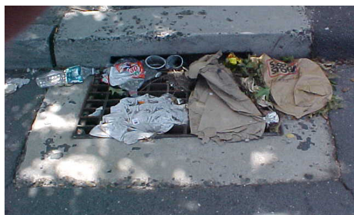
Figure 6. Typical mosquito breeding sites (top) clogged gutters around the home; (bottom) storm drain catch basin. (Photo Credit: (top) Purdue University and, (bottom) Centers for Disease Control and Prevention)
