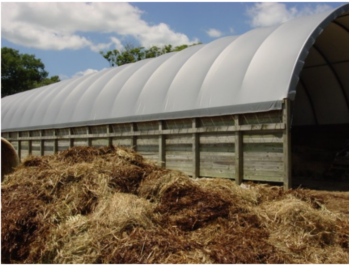
Hay in the foreground was removed from the hoop building because the hay was smoldering.
