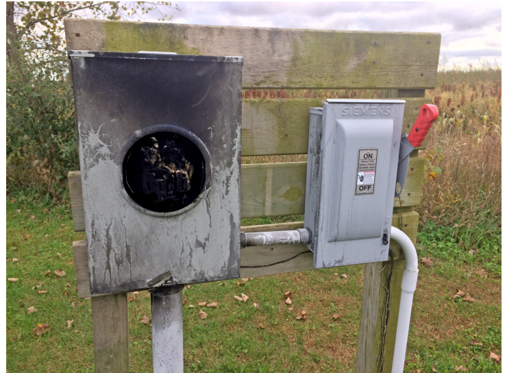
Lightning damage can result in the need for a total replacement of the metering unit and disconnect boxes. The sooner you find the problem, the more time you will have to replace it before irrigation is needed. Photo by Lyndon Kelley, MSU Extension.
