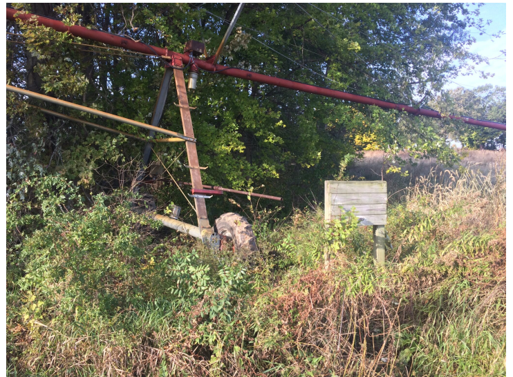
Stop control switches can fail, often due to waterlogged or freeze damage. Check the switch function and the alignment to the infield stop to avoid a run-away pivot. Photo by Lyndon Kelley, MSU Extension.
