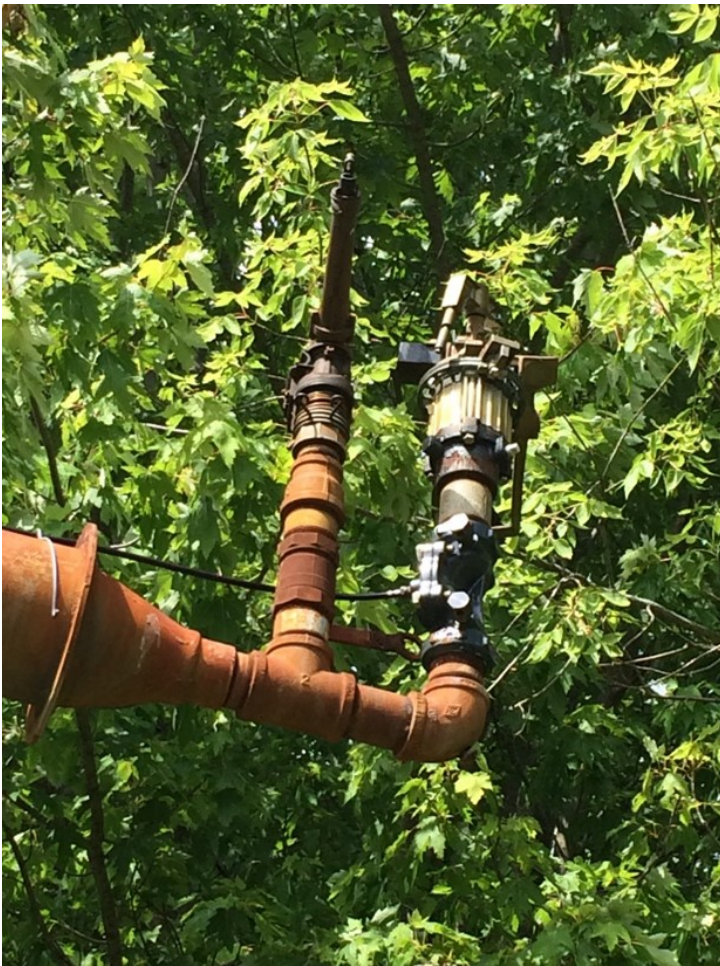
Unchecked fence row tree and brush growth into the path of the end gun and pivot end boom can create major damage. Photo by Lyndon Kelley, MSU Extension.
