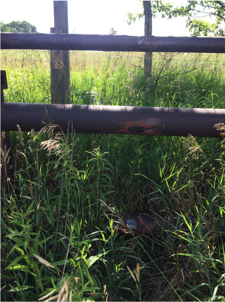
Tire wear marks on the stop barricade indicate the electronic stop has failed recently. Photo by Lyndon Kelley, MSU Extension.
