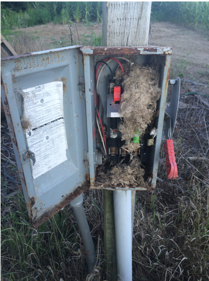
Vermin nests can cause explosions, electrical shorts and corrosion of wires. To avoid a dangerous situation, inspect and clean all electrical control boxes from the power supply to the pivot panel before energizing. Photo by Lyndon Kelley, MSU Extension.
